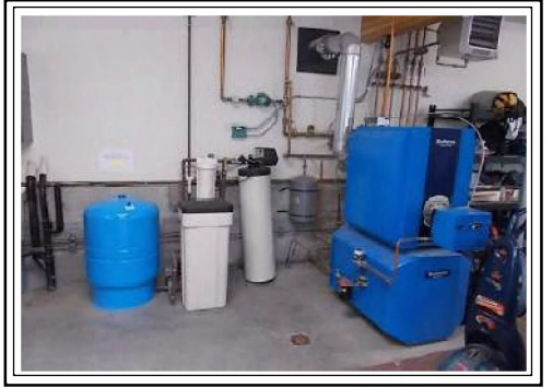
Mechanical in Garage
