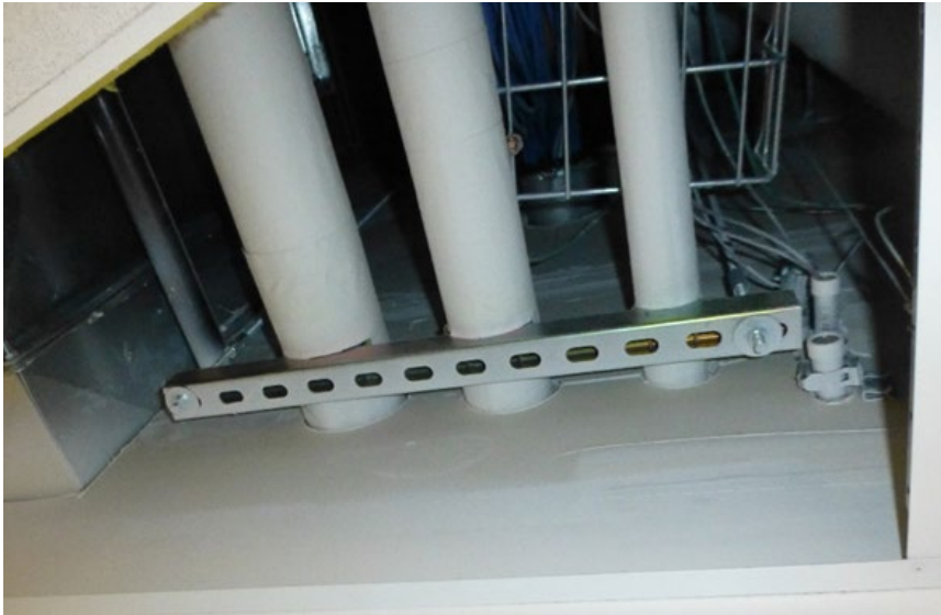
CW, HW, HWC piping above drop ceiling in corridor outside entry to boys' locker room. Piping with offset expansion loop is above hard ceiling and is concealed.
