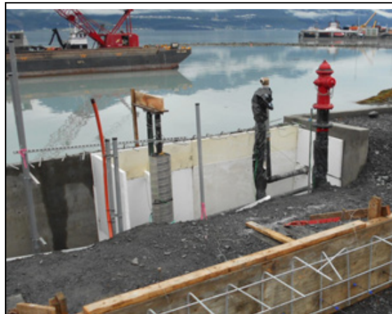
Insulating backflow preventer (BFP) foundation
