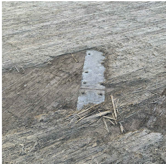
PHOTO #7 - WORN DECK WITH EXPOSED PLATE
