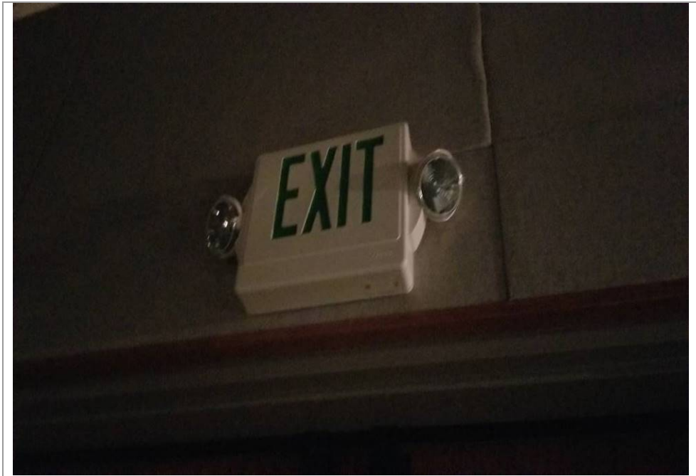
02-12219A: Civic Center (Theater); Replace batteries and lightbulbs to ensure emergency lighting activates in the event of a power outage.
