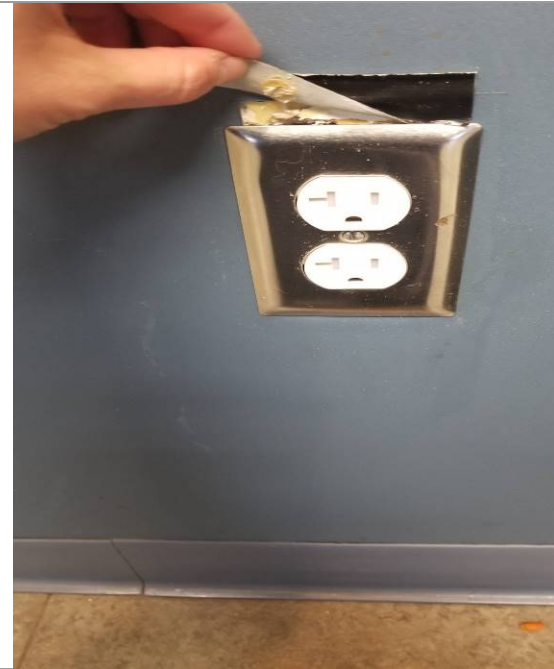
06-12219A: Rec Center, Fire Station; Repair broken electrical outlet cover to avoid arc flash, an electrical short, and live electrical exposure to employees and general public..
