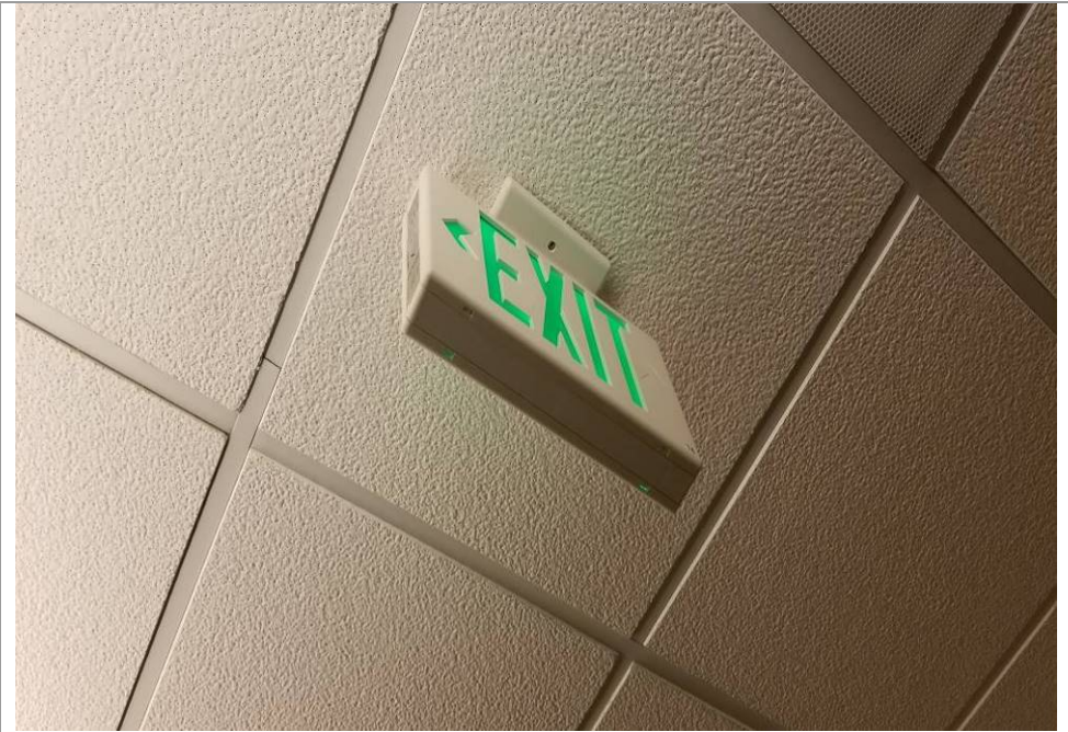
08-12219A: Hospital; Excellent new self-testing exit signs installed throughout the facility. Continue the good work!
