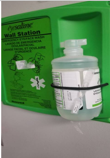
03-12219A: Civic Center (Kitchen, Janitor Closet); Expired eyewash solution. Recommend purchasing new eyewash solution.
