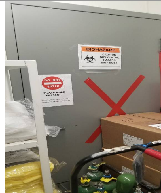
10-12219A: Fire Station (Throughout Building); The building was inspected 3 years ago and diagnosed with a severe type of black mold. As indicated by the picture, certain areas have been quarantined due to black mold. Staff continue to work around the quarantined areas and state they feel sick after a day of work. During my inspection at this facility, I immediately experienced a headache that dissipated after I left. On May 6, 2019, the Valdez city council voted no on a proposal to relocate and construct a new fire station.
