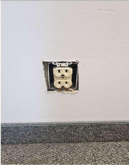
09-12219A: Police Station (Stairwell); Replace broken electrical outlet cover to avoid arc flash, an electrical short, and live electrical exposure to employees.
